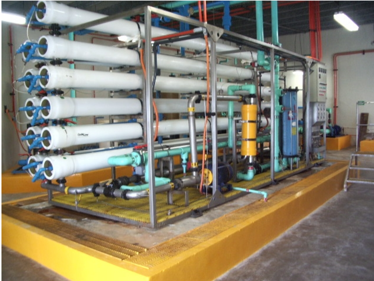
Reverse Osmosis Water Purification System 700-room Resort Hotel
